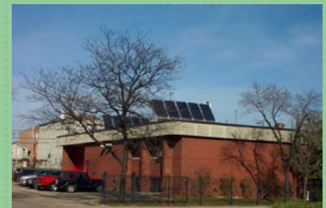
Solar thermal installation
